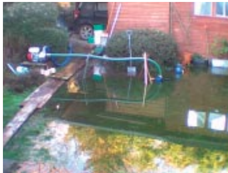
A submersible pump in operation
